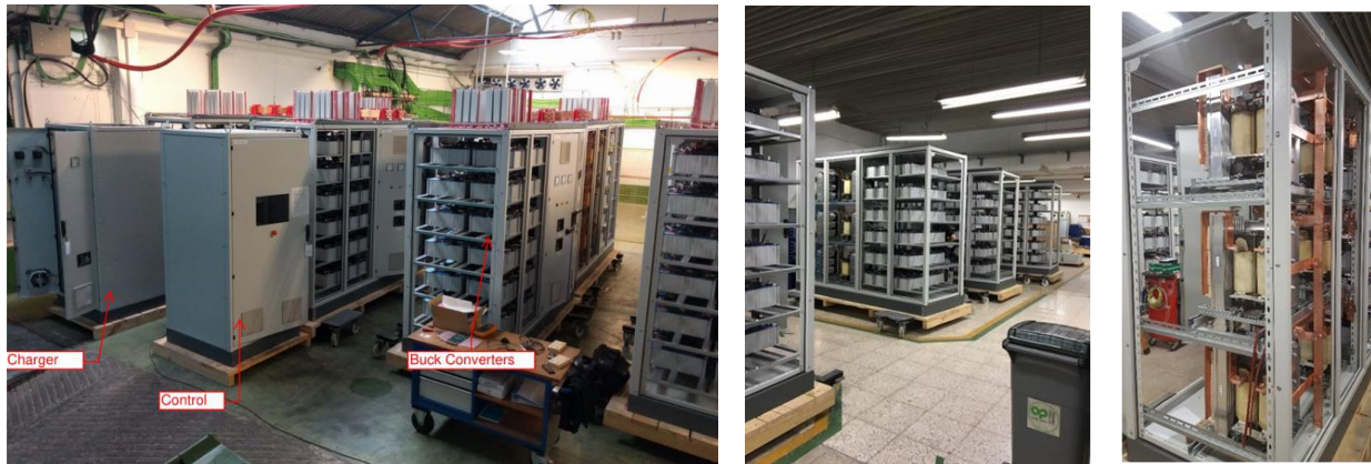
FIG.9. Power supply units.
