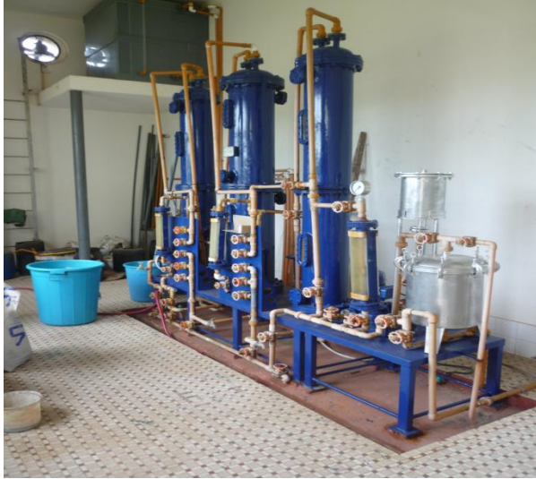
Fig 3c. Old deionized water plant
