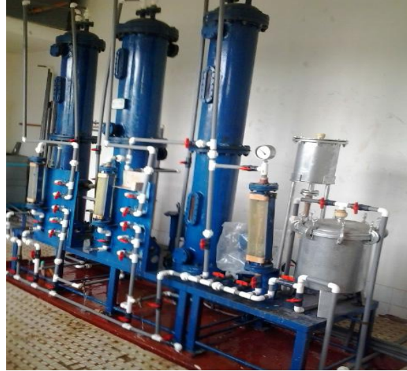
Fig.3b Refurbished deionized water plant
