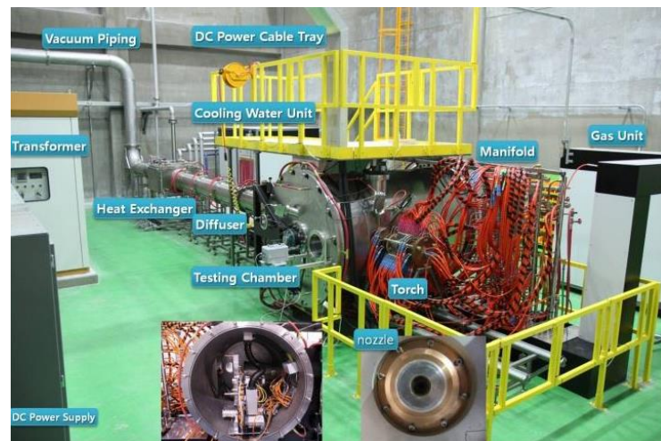
2.4 MW PSI Test Facility
