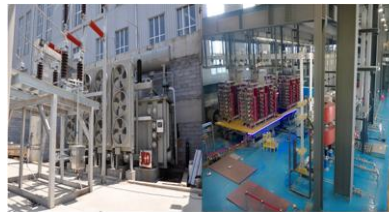
System Integration of the PFCU at ASIPP site
