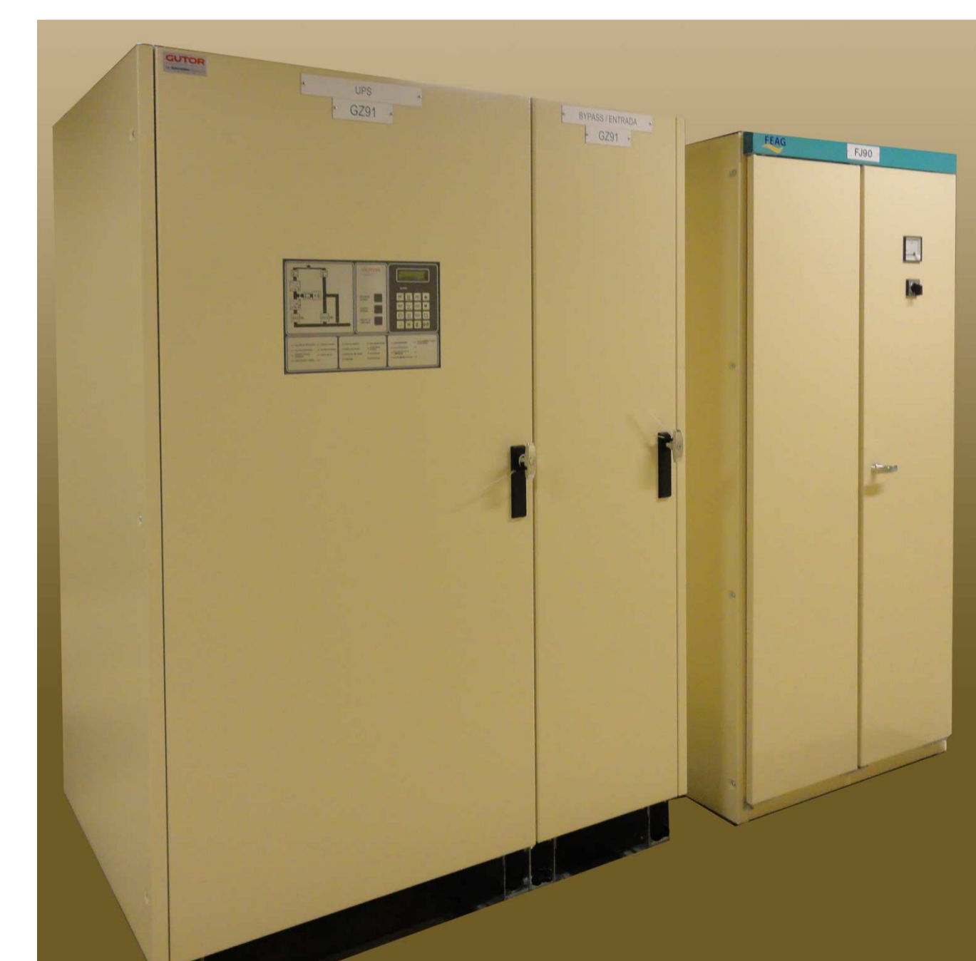
Figure 5: Electrical Cabinets and Battery Rack
