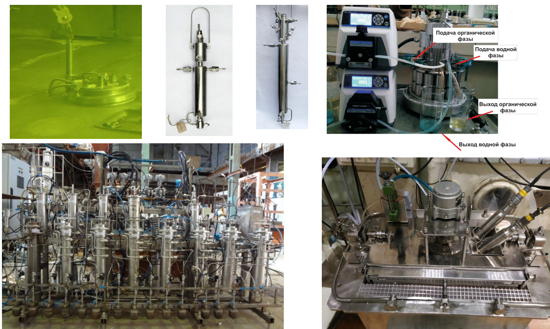
Figure 6. Dissolution, extraction, gas purification and actinide oxides preparation facilities
