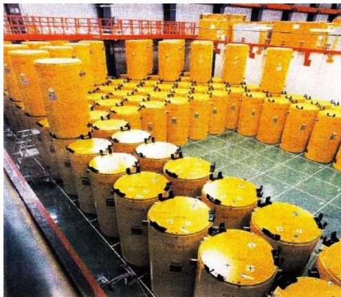
CASK DRY STORAGE
