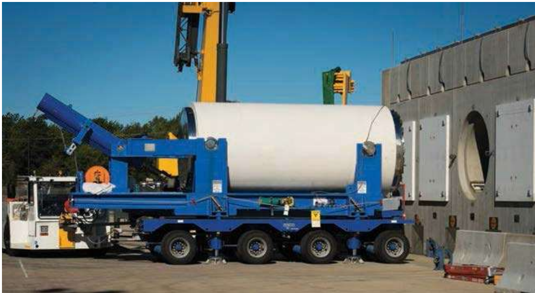
FIG. 1. External view of ANPP SNF dry storage facility.
