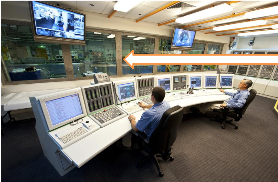
OPAL Reactor Control Room
