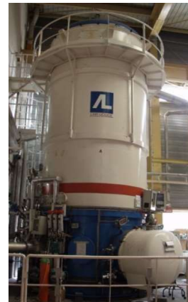
FIG. 3. WEST Cold box
