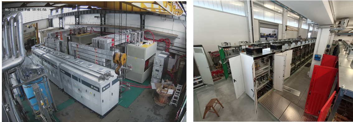
FIG. 5. A) Image of the FCCT facility where the DTT TF power supply has been temporarily assembled and commissioned. B) Image of the 27 cabinets manufactured for the 27 independent power supply of the non-axisymmetric coils at EEI.
