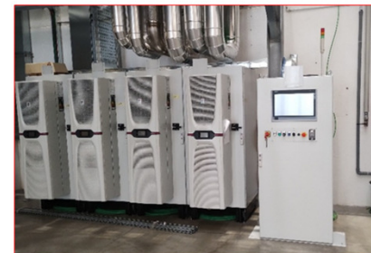
DC Power Cabinets and Control Units (tested in May 2024)
