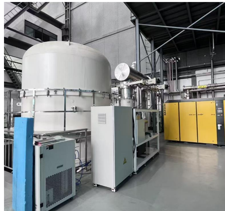
Thermal-Hydraulic test platform (D3m*H6.2m, 4.5K@200W)
