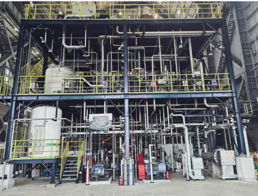
Supercritical CO 2 loop for thermal hydraulic testing
