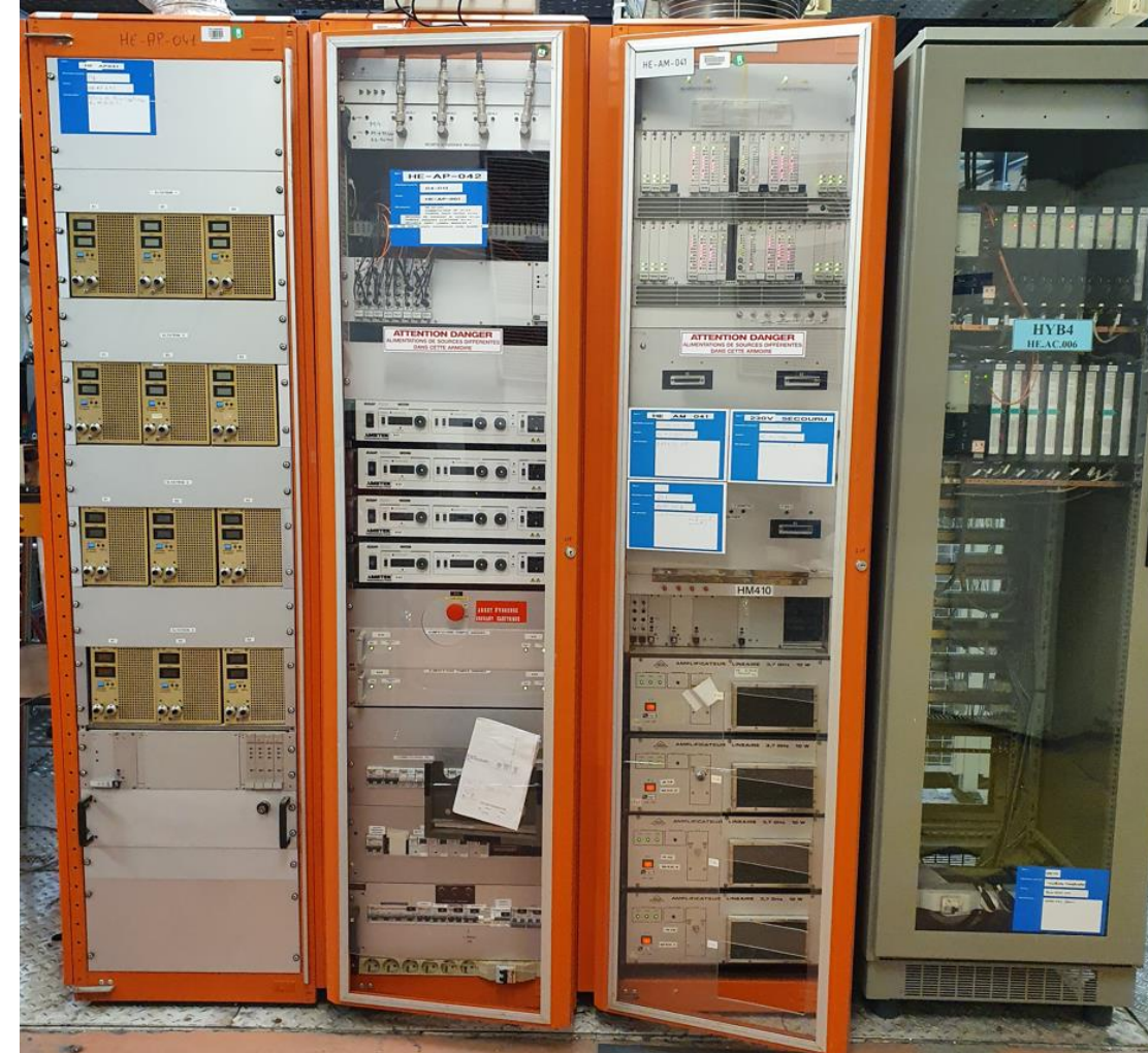
Racks for one module of 4 klystrons
