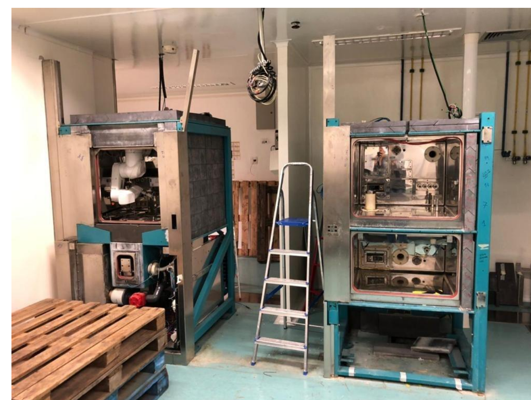
Figure 2: Hot cell dismantling during the decommissioning step in Cyclotron facility in Brazil (CNEN collection)
