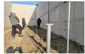
Measuring sensor installation
