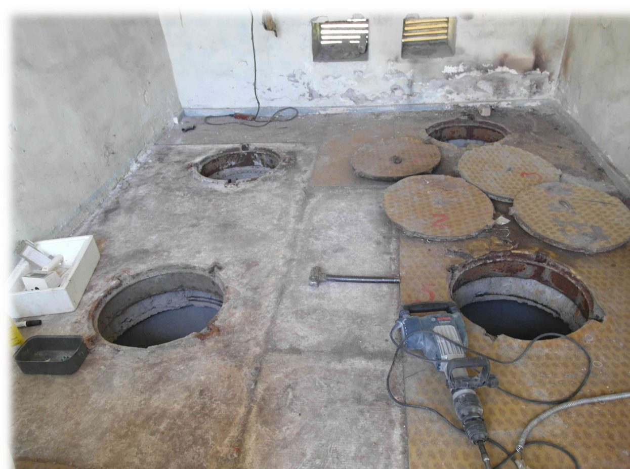
Decontaminating wells in isotope storage building
