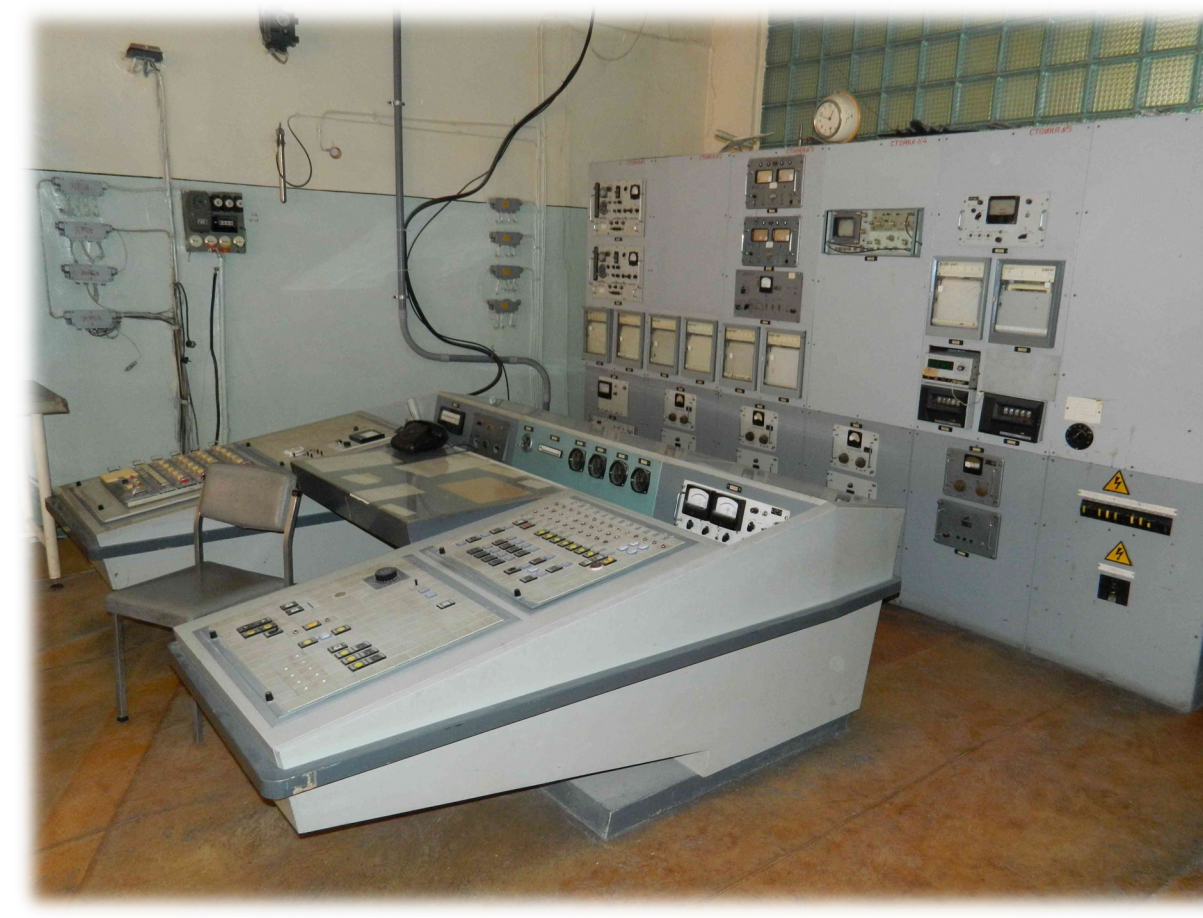
IIN-3M reactor control panel
