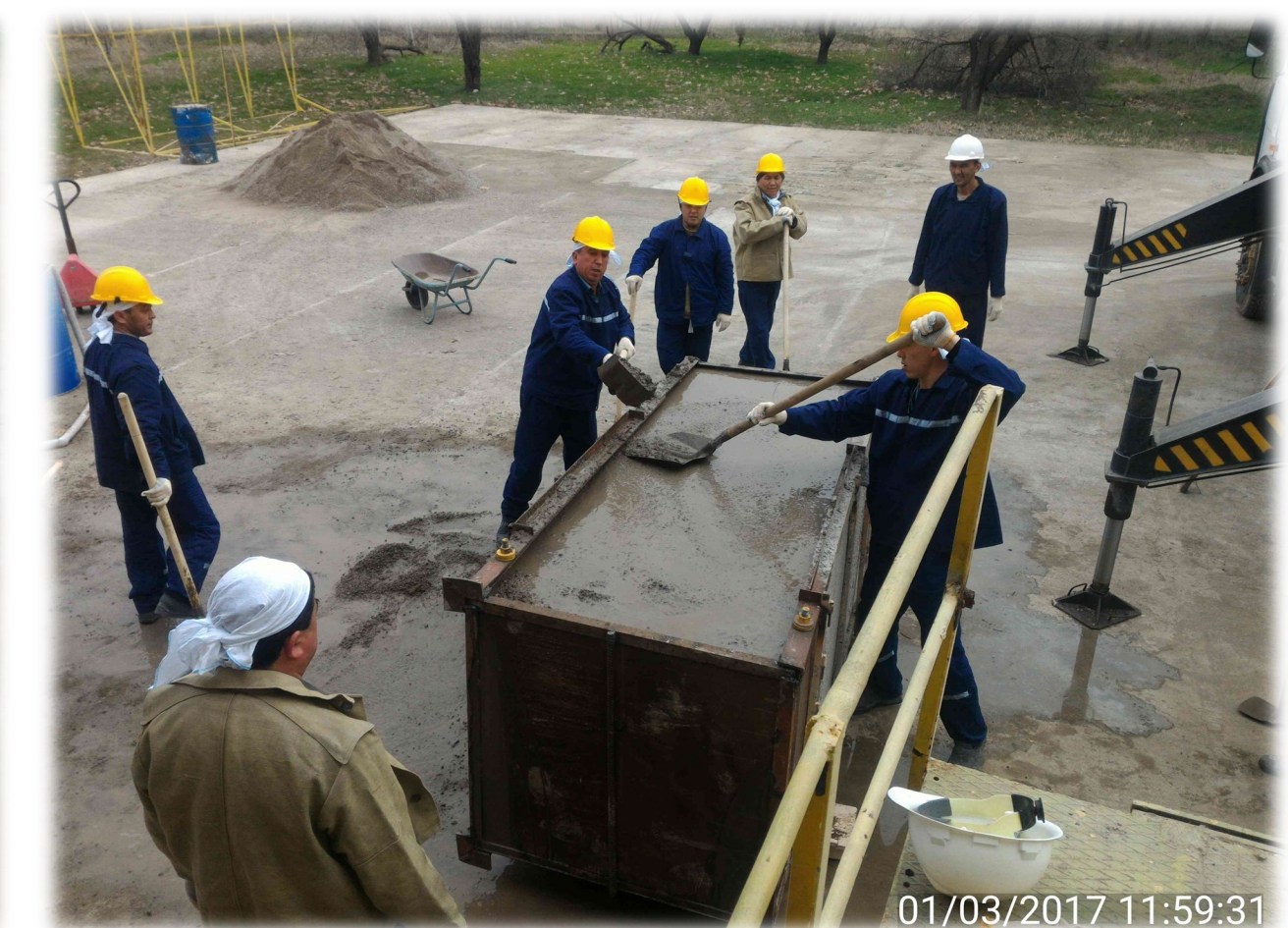
Reactor vessel in a container with concrete
