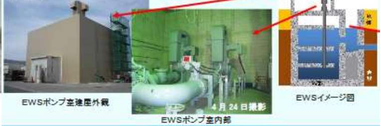
EWS Pump Building
