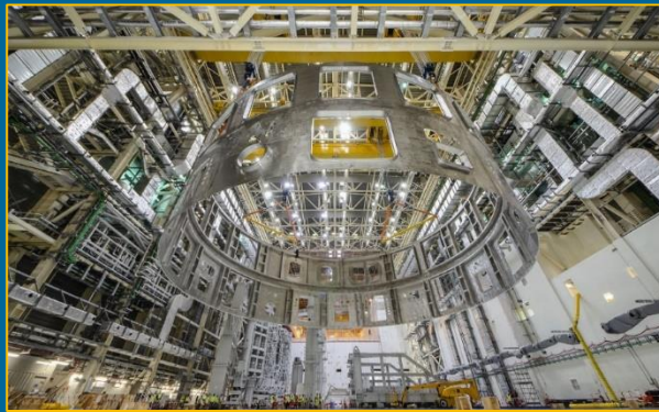
31 Aug 2020 - Cryostat Lower Cylinder
