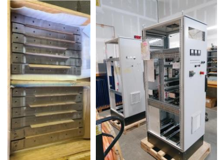
Support Structure & Power Supply
