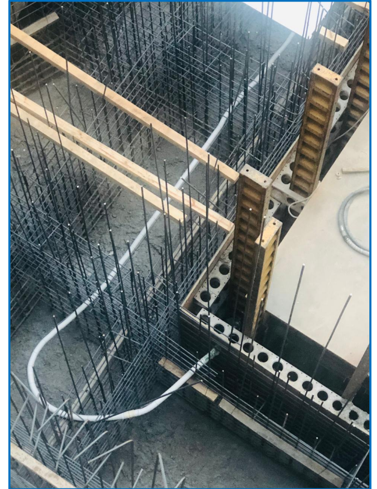
Absence of intern metallic tensors
