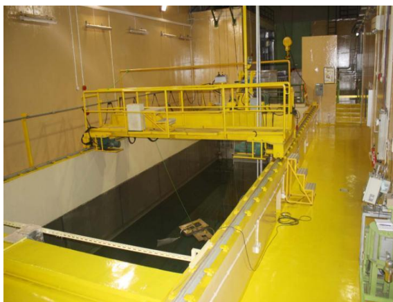
Fig.4. Spent Fuel Interim Storage
