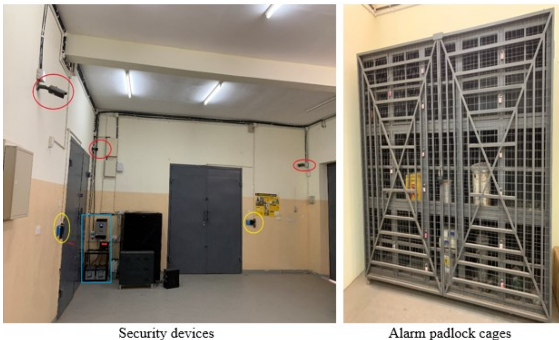
Fig. 3. Security systems inside the radioactive source storage facility
