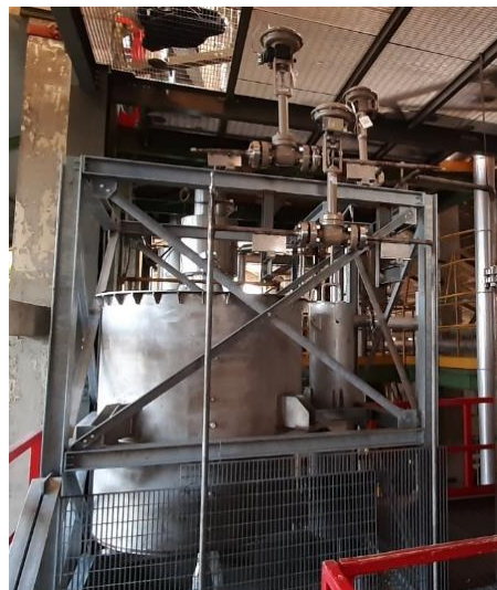
FIG. 17. SIRIO cooling system.
