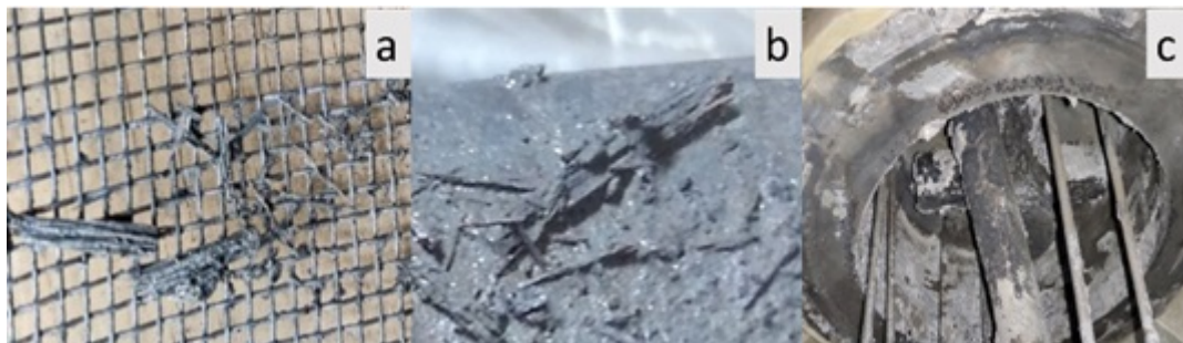
Figure 1: Figure 1: Deposition of corrosion impurities on the surface of a) CT wire mesh packing and b) CT outlet pipe, c) deposition of oxide impurities on interior walls of CT
