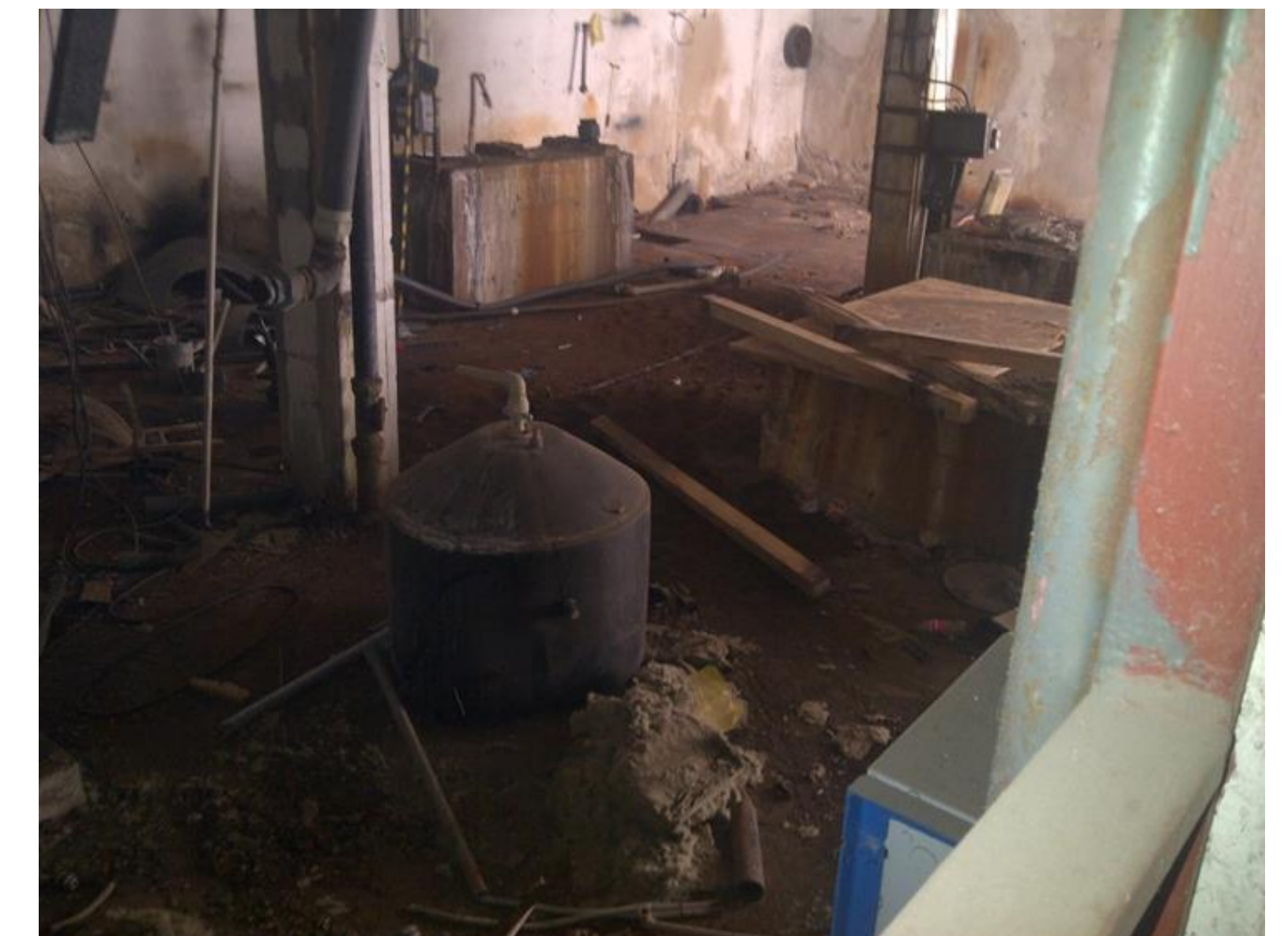
Fig.3. NORM workplace Water treatment plant of public swimming pool in reconstruction
