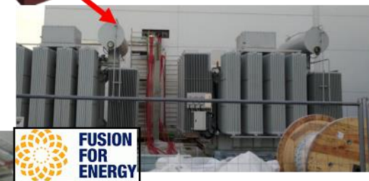
Fig. 15. AGPS Conversion system 60MW CW
