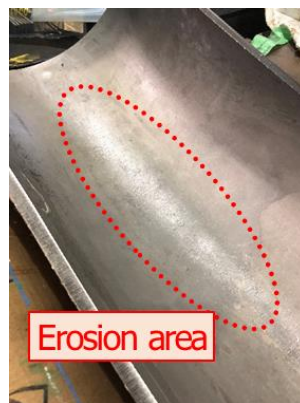
FIG. 8 Discoloration area inside the downstream conduit after disassembly of ELTL
