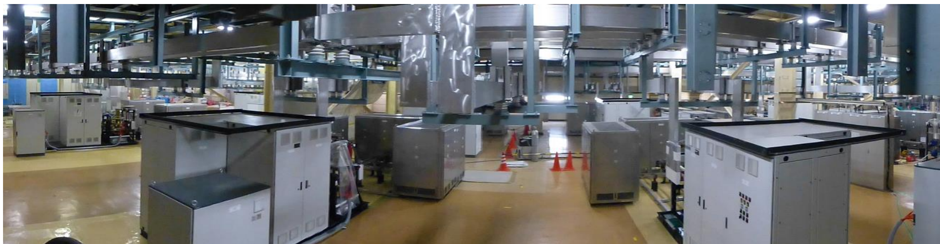
Panoramic view of some Quench Protection Circuits after installation in one JT-60SA Power Supply hall
